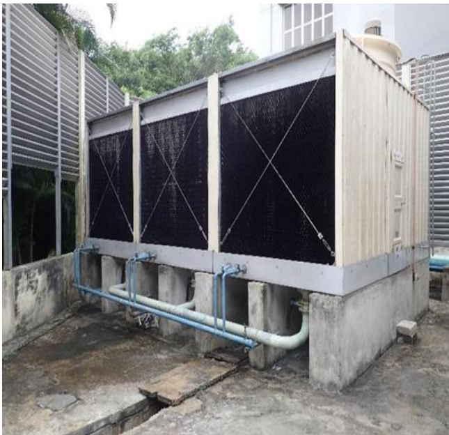
Perdanasiswa Complex (KPS) Cooling System
