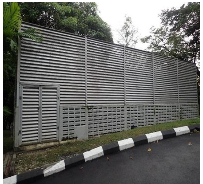
Tunku Chancellor Hall (DTC) Cooling System
