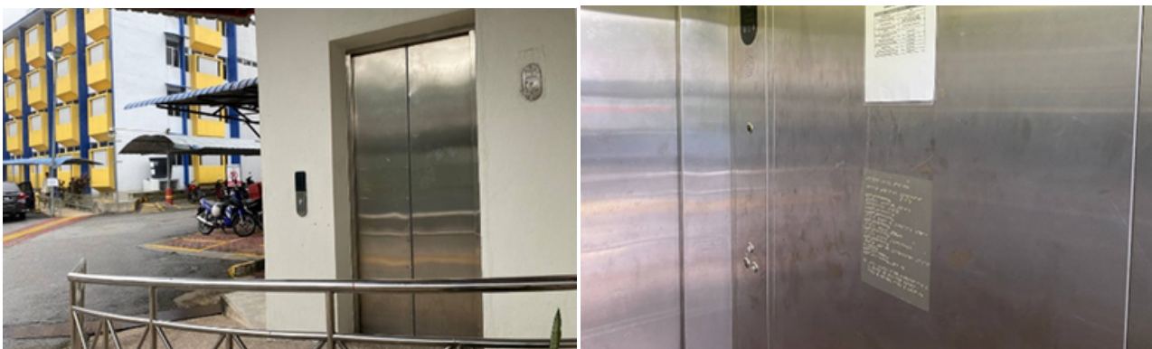
Below: An elevator at Kolej Kediaman Ketujuh (Za'ba) featuring Braille signage, making it easier for individuals with visual impairments to navigate the building independently
