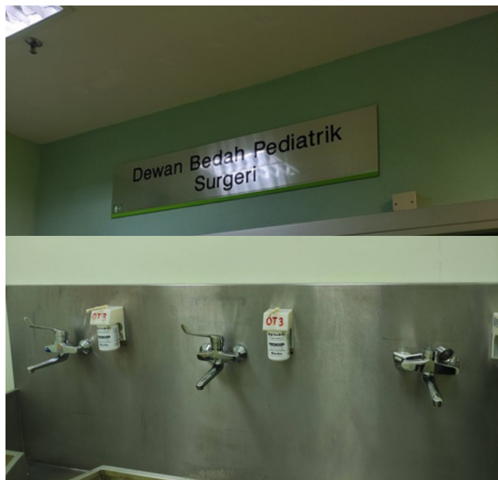
Above: Water taps at Dewan Bedah Pediatrik, UMMC, fitted with tap aerators to reduce water flow
